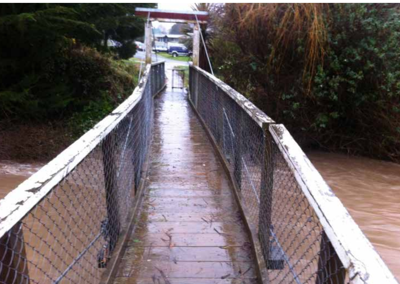
Figure 11: Erne Street foot bridge (Waitati), damaged after the 2017 floods. Photo: BRCT / Scott Willis
